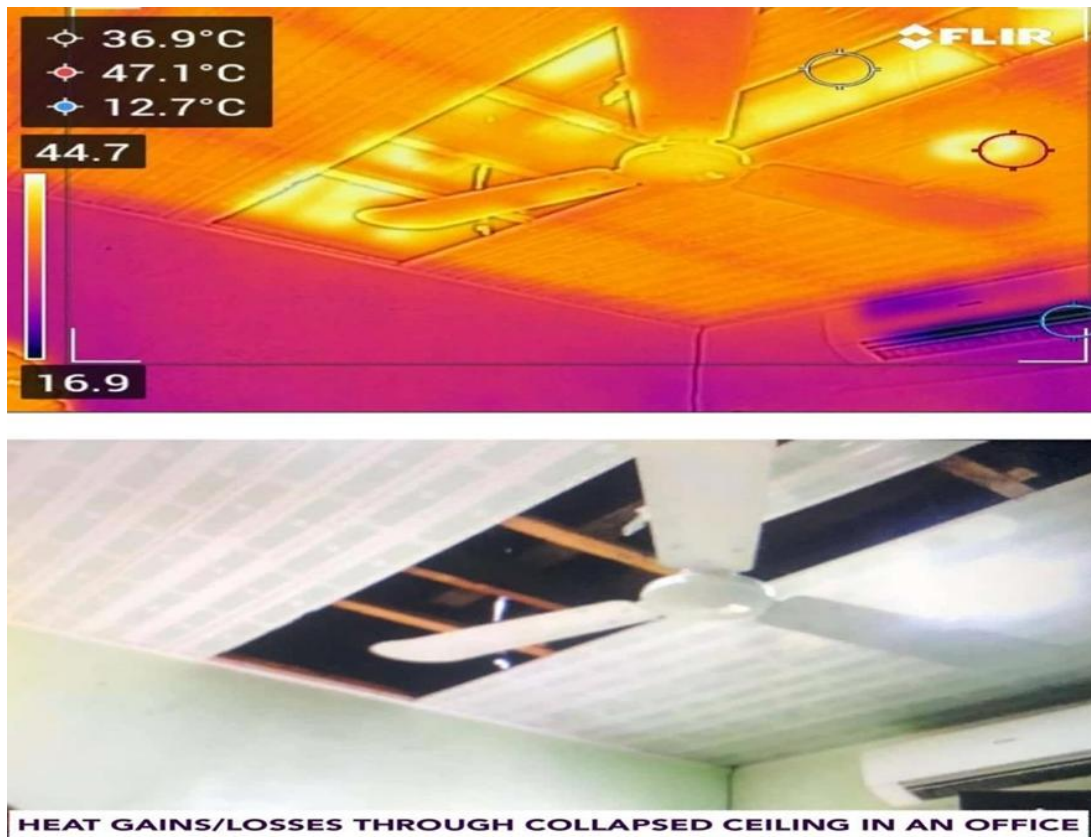
Figure 14. Heat Gains and Losses Through Collapsed Ceiling of an Office
