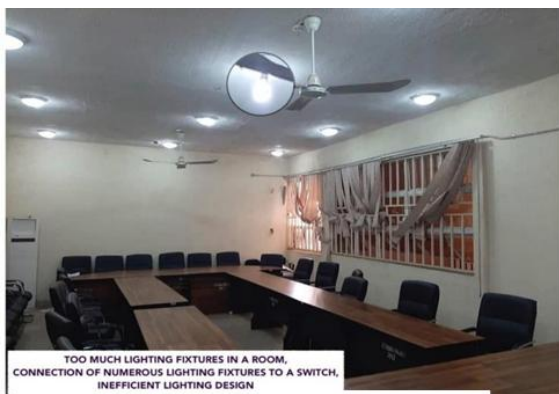
Figure 7. Improper Light Fixtures in a Room
