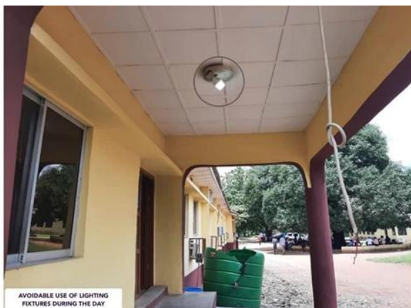
Figure 8. Avoidable Use of Light Fixtures During the Day
