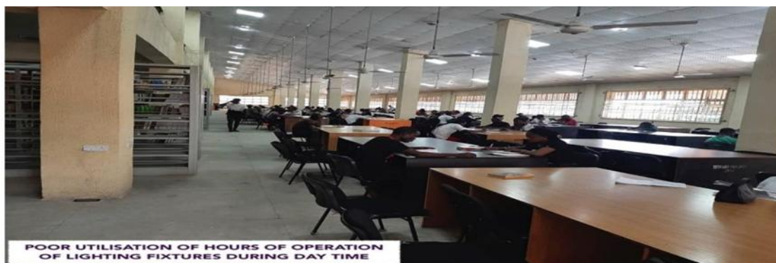
Figure 9. Poor Utilization of Hours of Operation of Light Fixtures During Daytime
