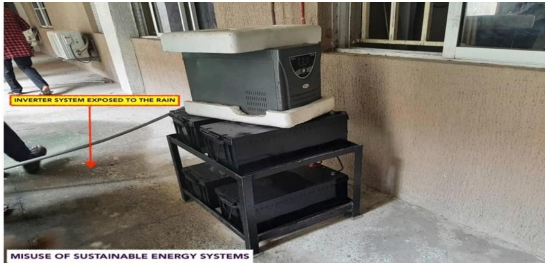
Figure 15. Misuse of Energy System
